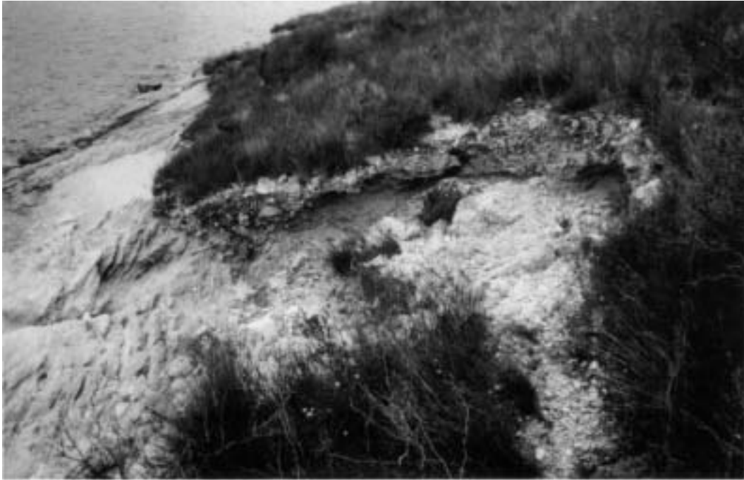
Figure 10: Small landslide on reservoir perimeter west of Scotts Peak Dam, caused by wave erosion removing toe support from slope deposits. Slope failures of this kind appear uncommon around this reservoir (photo: K. Kiernan).
